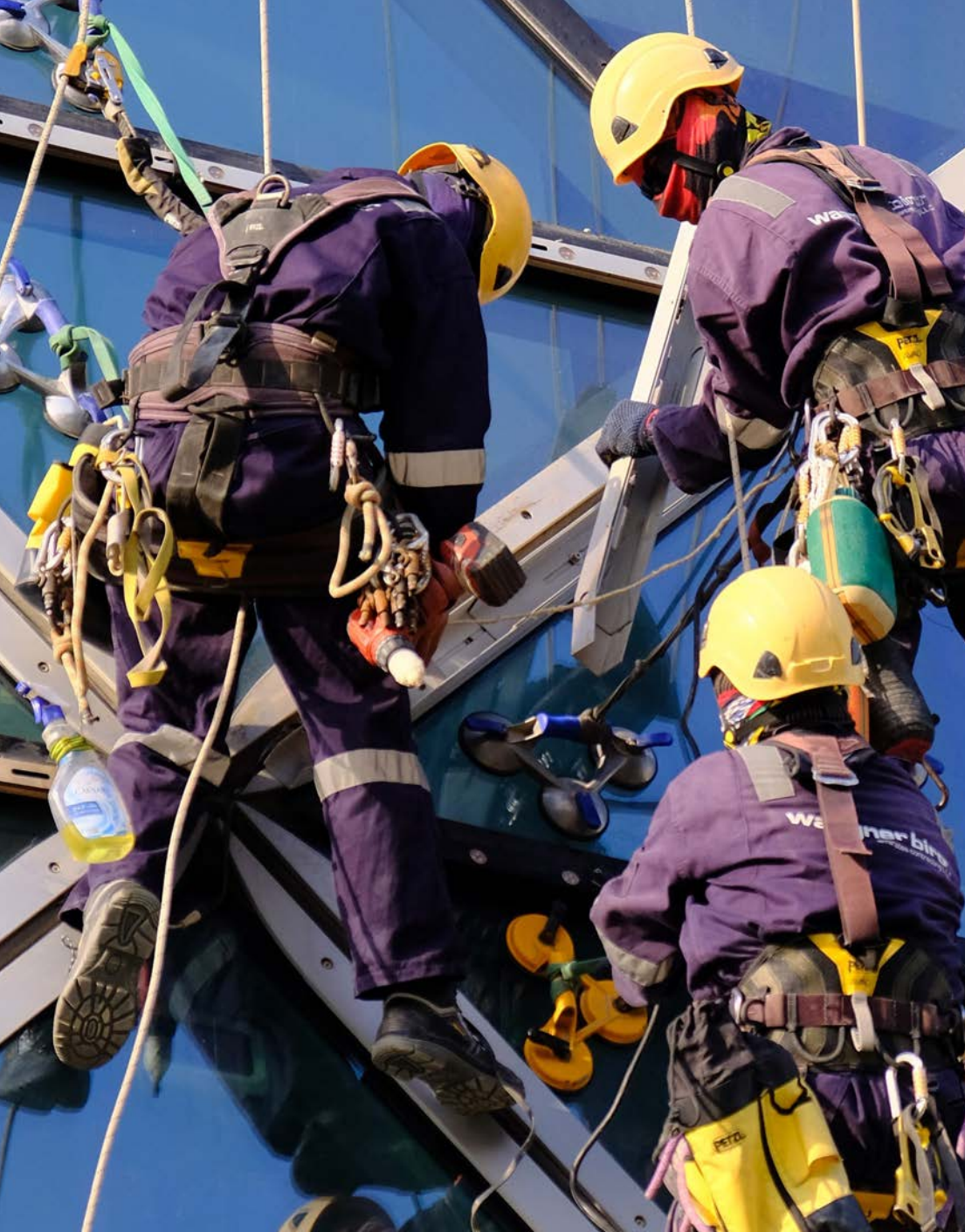
Adnec Tower/Capital Gate: Installing LED-strips by façade climbers trained for highest occupational safety.
