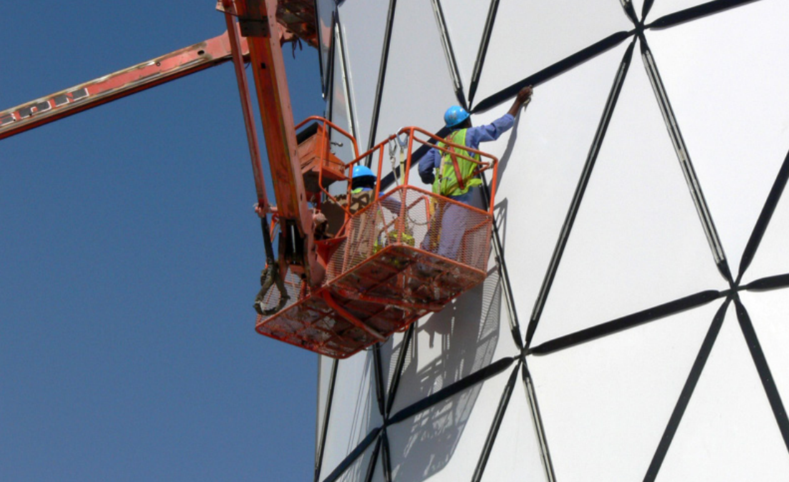
Sun Tower, Yas Marina Formula One Racing Circuit, Abu Dhabi: Façade cleaning works
