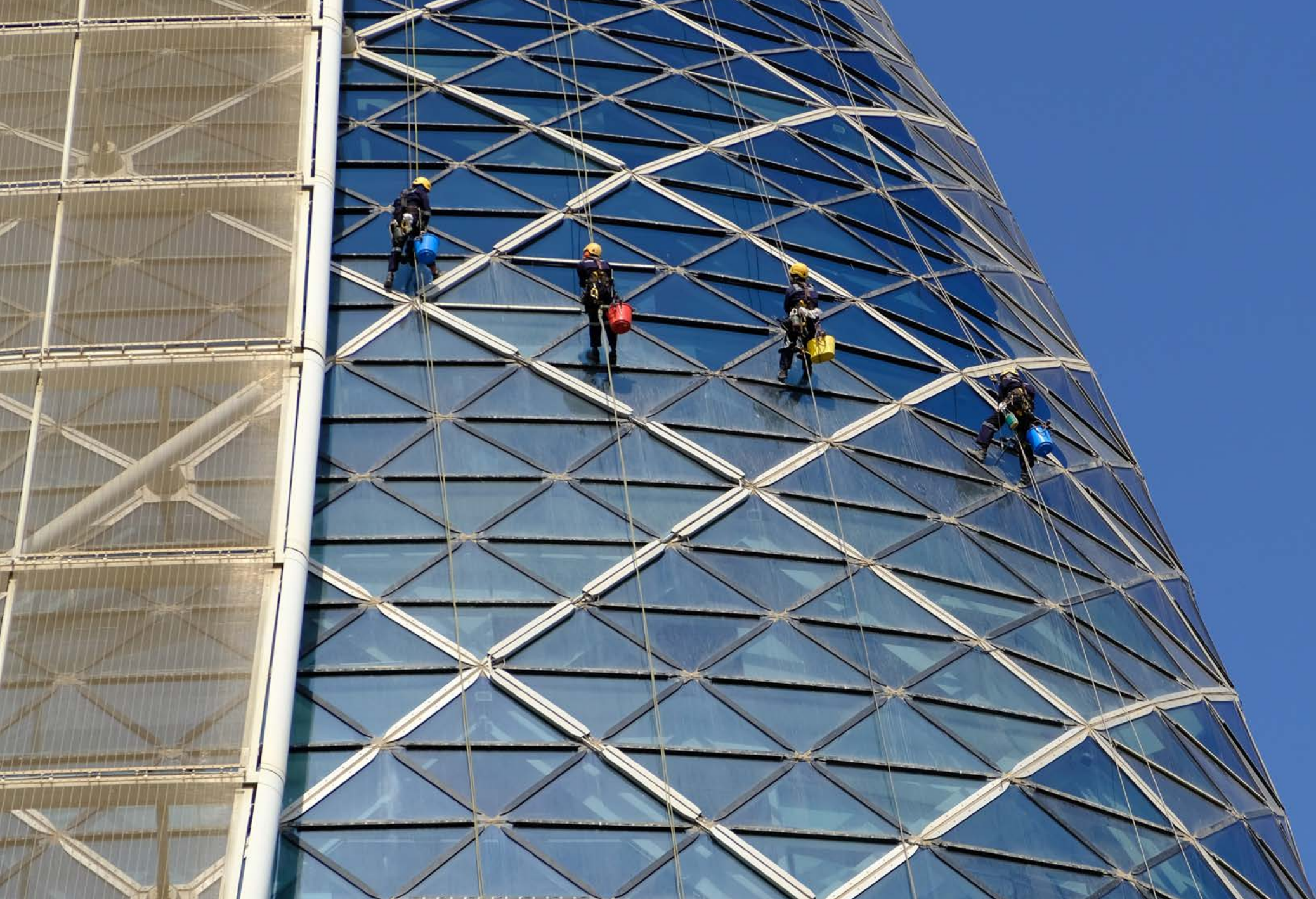
Adnec Tower/Capital Gate, Abu Dhabi: Our team of specialist rope access technicians in cleaning action
