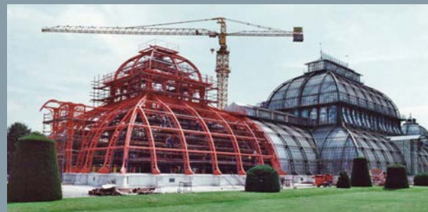
In 1991 Waagner Biro won the European Steel Design Award for the outstanding efforts on renovating the “Palmenhaus”.
